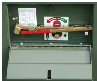
Switch-Operating Handle Storage
